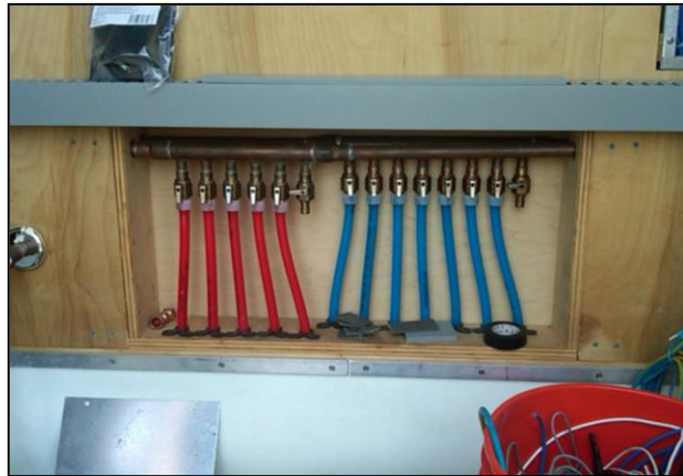
The University of Maryland WaterShed house features red and blue Uponor AquaPEX® tubing and ProPEX® fittings for the hot and cold potable plumbing system.
