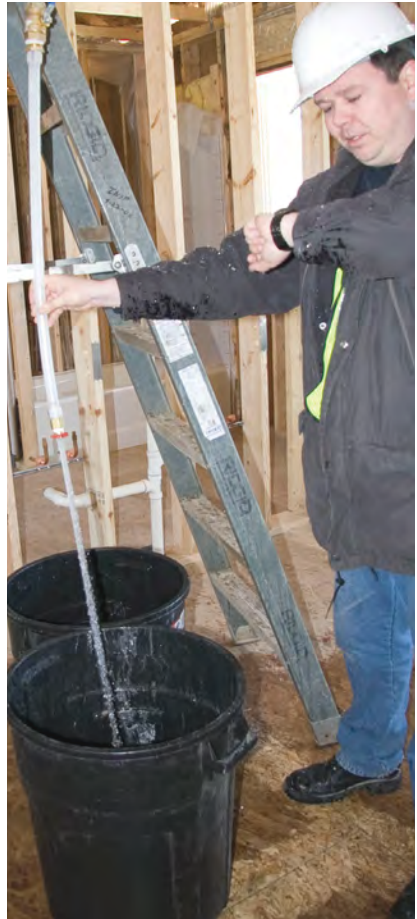
Figure 11-1: AquaSAFE flow test
